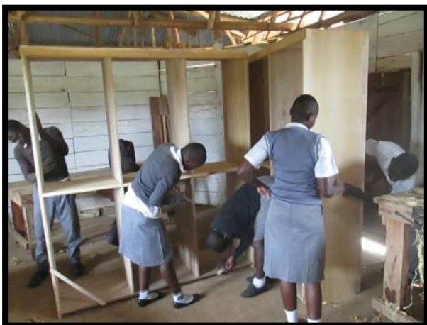
Students started building the cabinets in Sept. Cabinets were built for each of the 12 Boys' / Girls' huts by the High School Students
