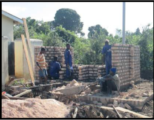
New Pit Latrine for Primary School under construction to be ready Feb. 2, 2015.
